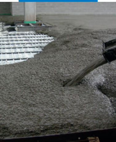
Pouring concrete with the addition of Mapecibre NS12 to counter plastic shrinkage
